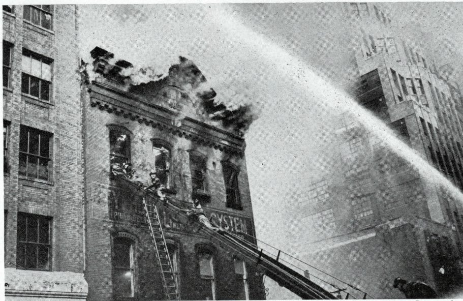
NO EXEMPTIONS FOR OLD AGE — The date on the front of this blazing loft building bears testimony that it had been standing unscathed for 89 years
